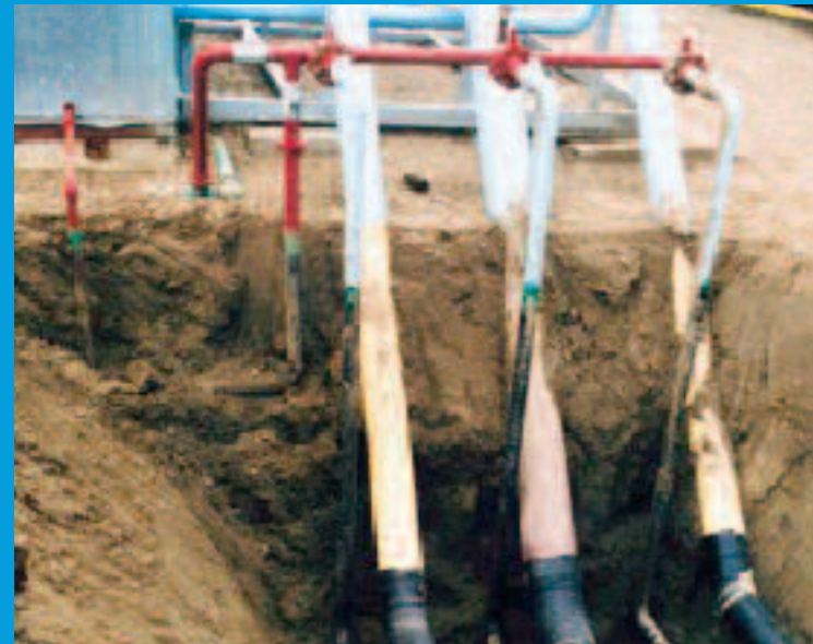
Live Gas Lines Exposed
